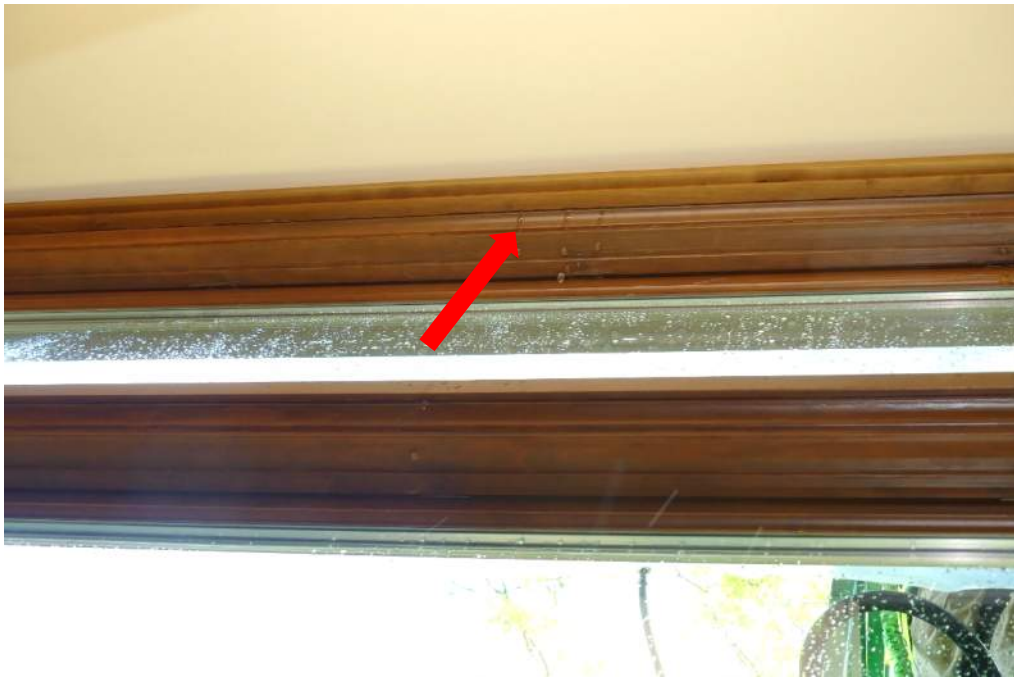
Photo 22 – Leak emanating between frame and trim
