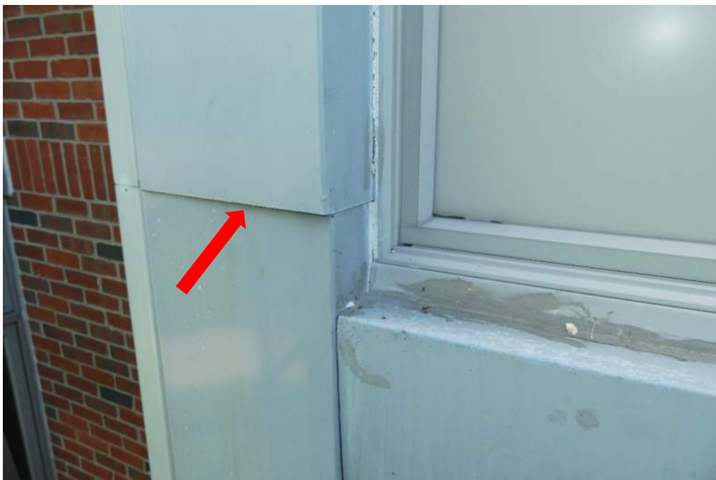
Photo 4 – No sealant at column cover splice
