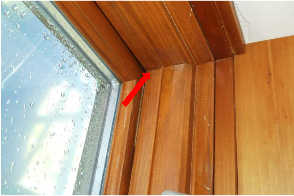
Photo 21 – Leak emanating between frame and trim
