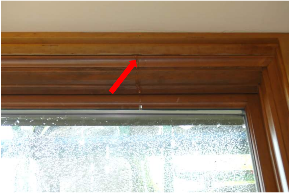
Photo 19 – Leak emanating between frame and trim
