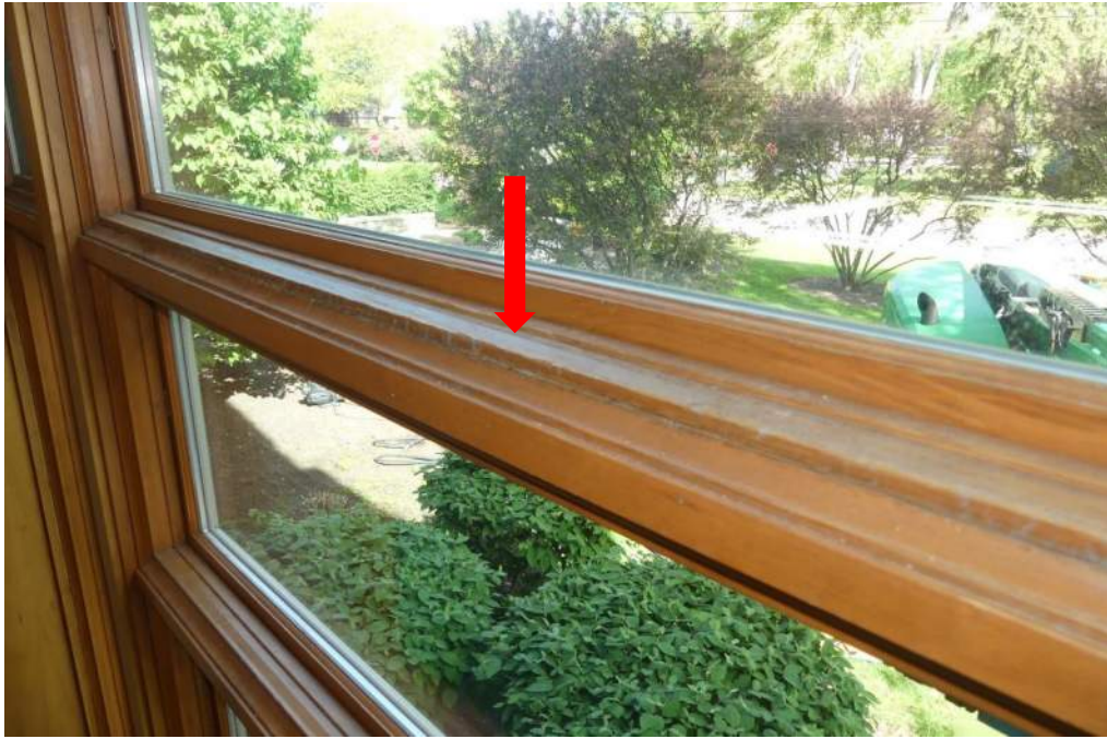
Photo 9 – Evidence of prior water leakage
