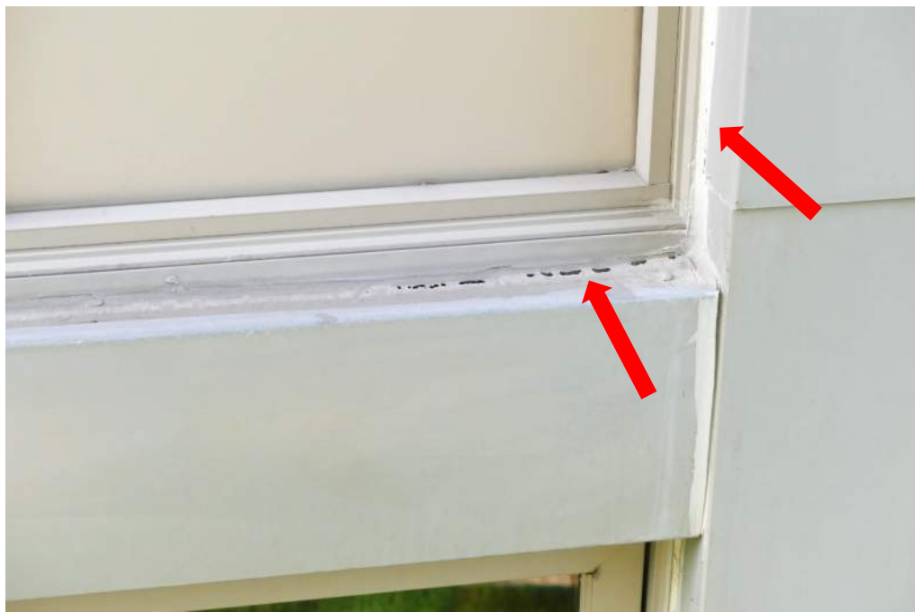
Photo 2 – Sealant exhibiting cohesive failure
