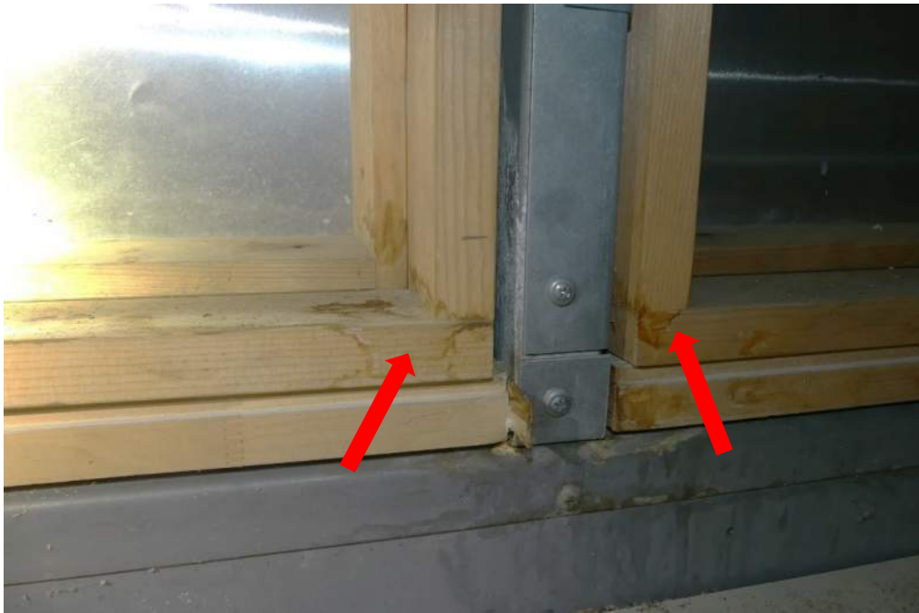
Photo 12 – Evidence of prior leaks on wood framing
