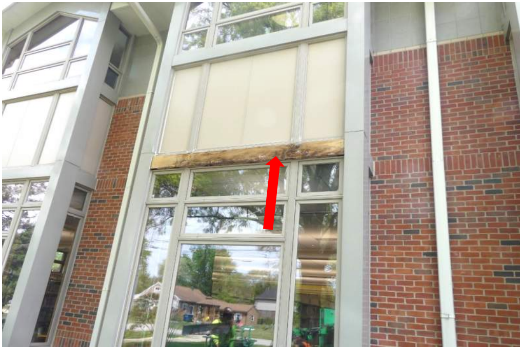
Photo 26 – Plywood sheathing exhibiting evidence of prolonged exposure to moisture
