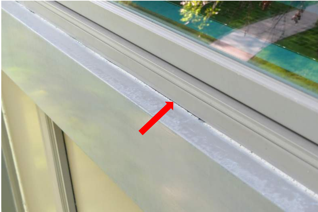
Photo 3 – Sealant exhibiting cohesive and adhesive failure
