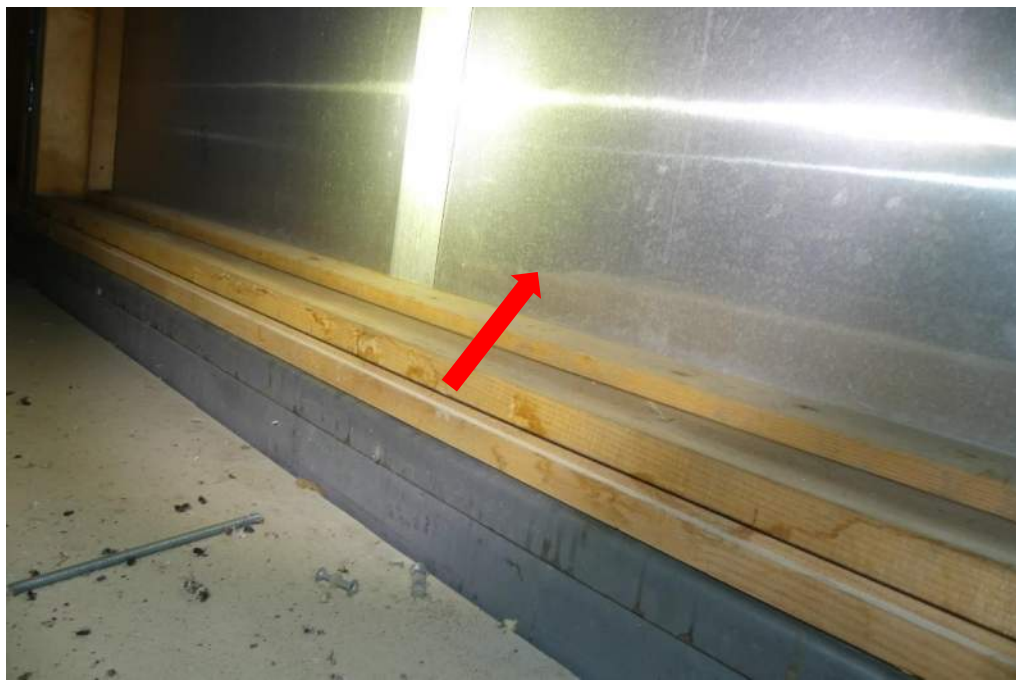
Photo 14 – No insulation or air barrier behind spandrel panels
