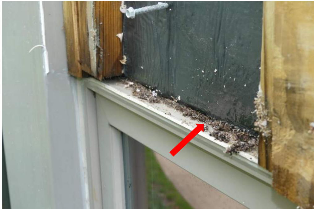
Photo 28 – Debris along top of window
