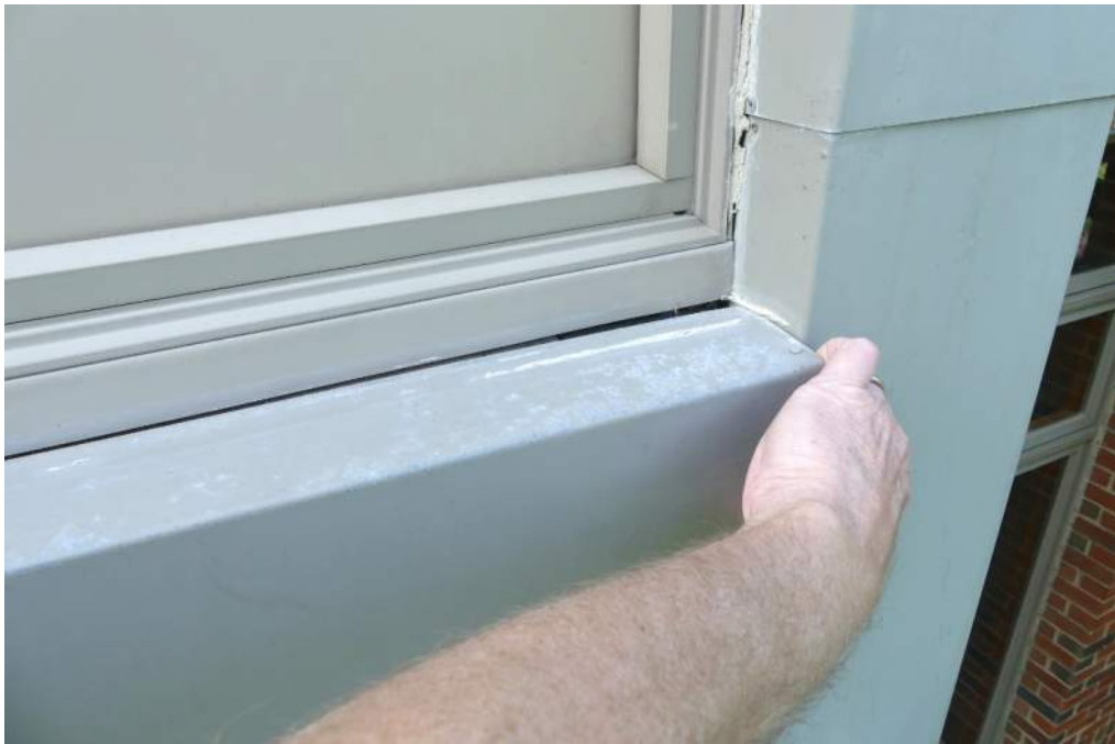
Photo 6 – Loose sill cover
