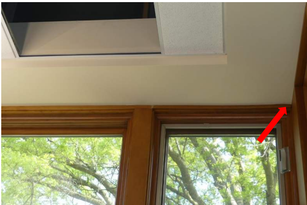
Photo 8 – Evidence of prior water leakage
