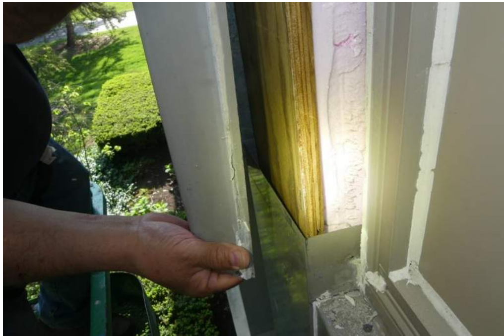
Photo 32 – Column cap pulled back
