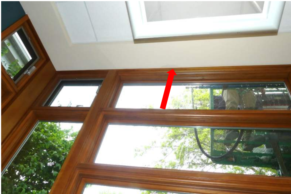
Photo 10 – Evidence of prior water leakage
