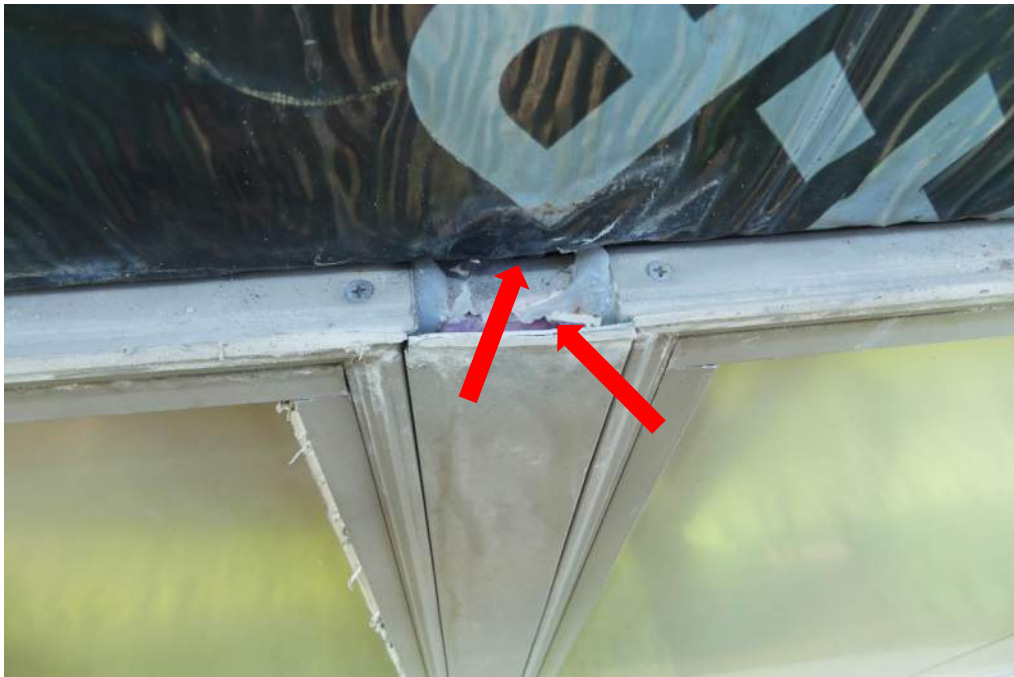
Photo 30 – Openings in top of mullion cap
