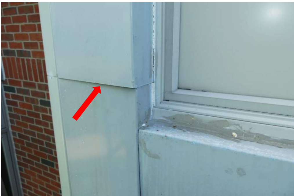
Photo 4 – No sealant at column cover splice
