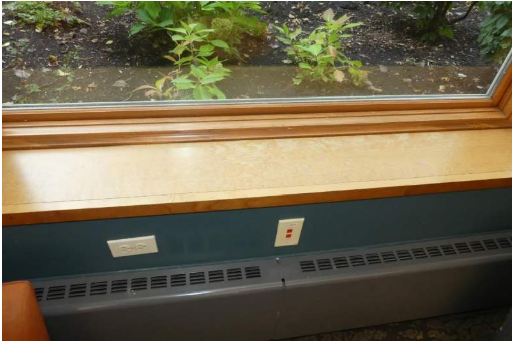
Photo 7 – Evidence of prior water leakage
