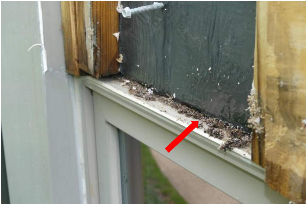
Photo 28 – Debris along top of window
