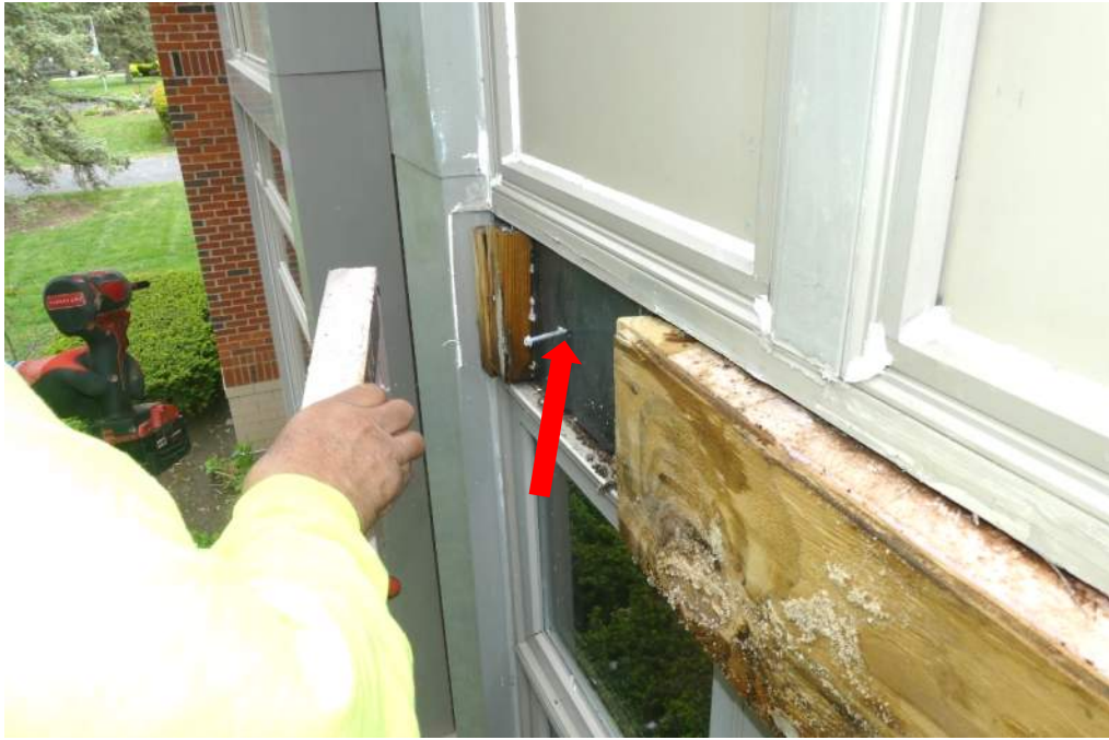
Photo 27 – Screw through insulation
