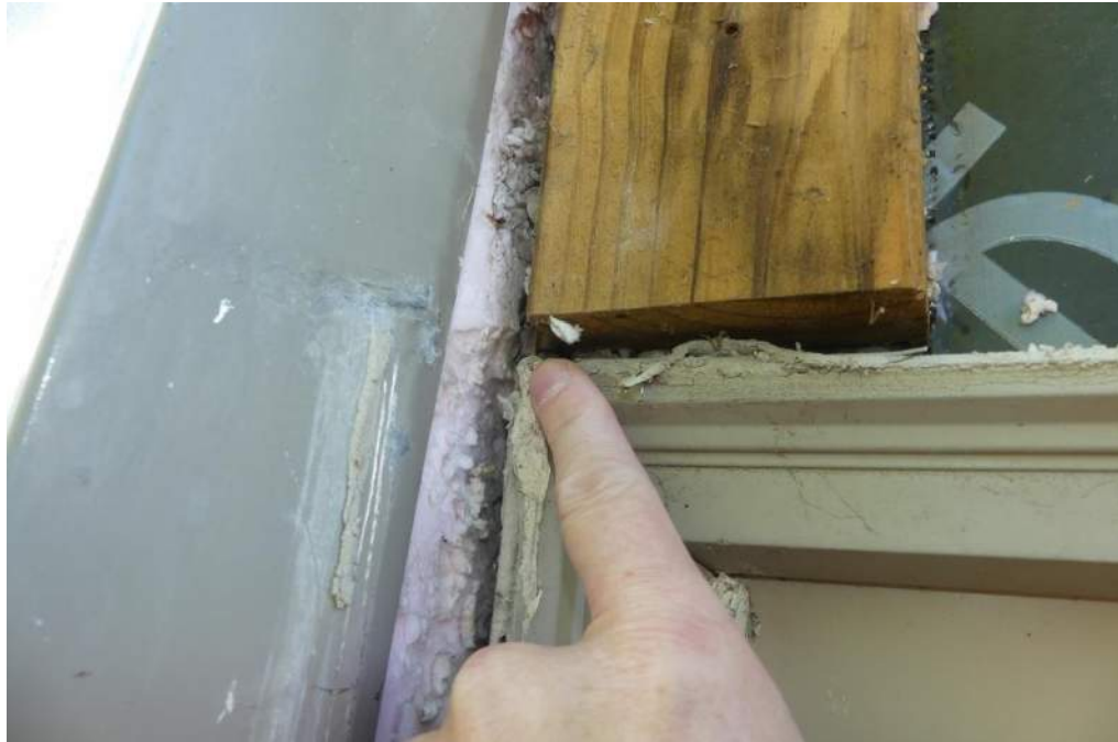
Photo 33 – Open joint between spandrel panel and vertical framing
