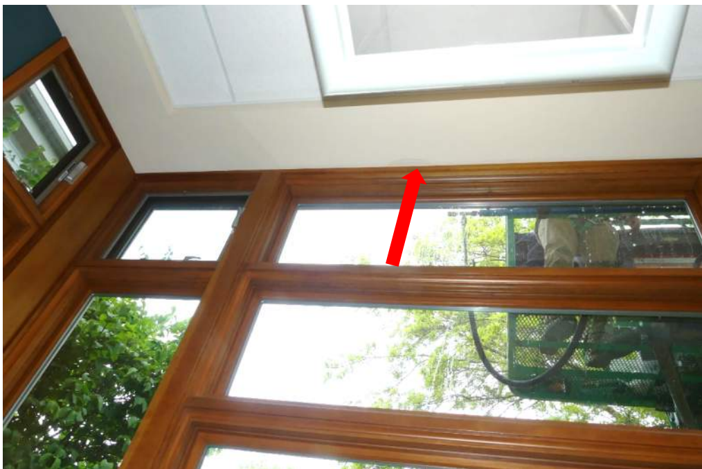
Photo 10 – Evidence of prior water leakage
