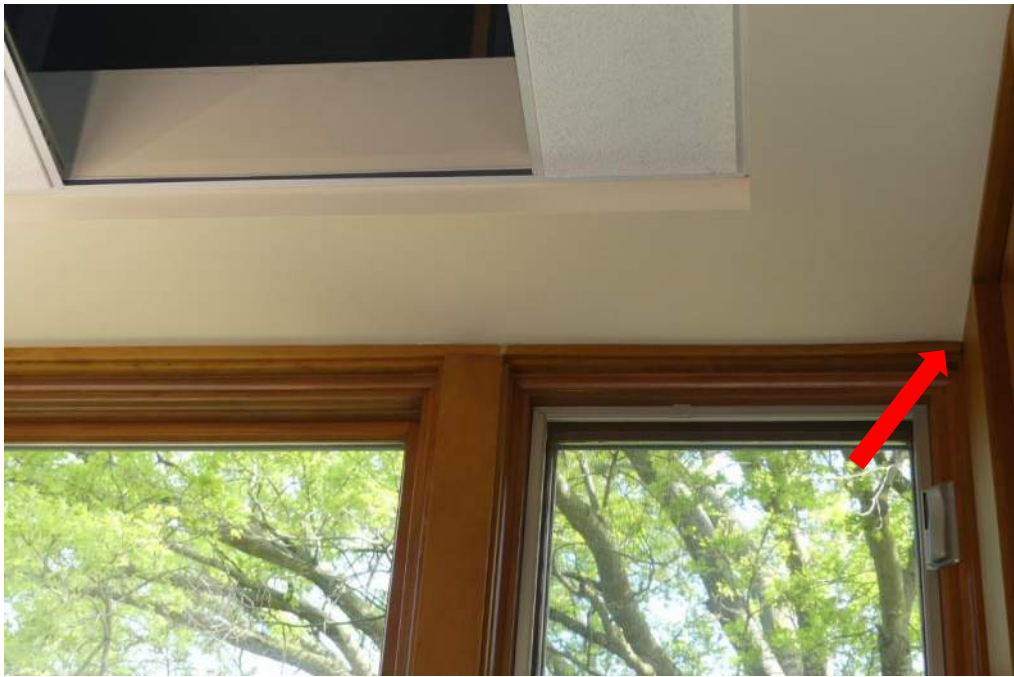
Photo 8 – Evidence of prior water leakage
