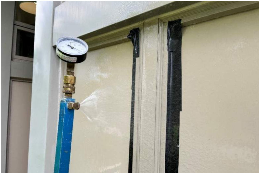
Photo 16 – Modified spray rack water test
