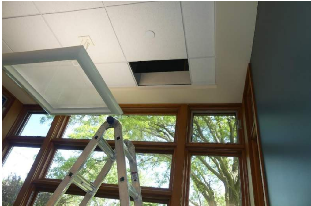
Photo 11 – Ceiling tile removed at middle bay
