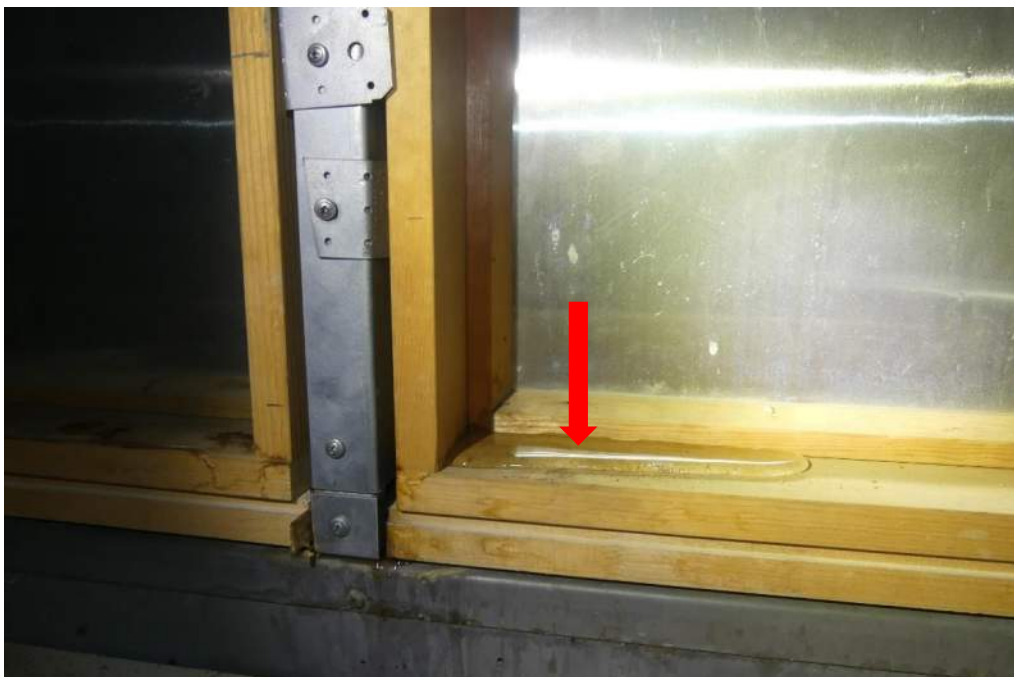
Photo 24 – Leak observed during test along 2 nd floor window sill
