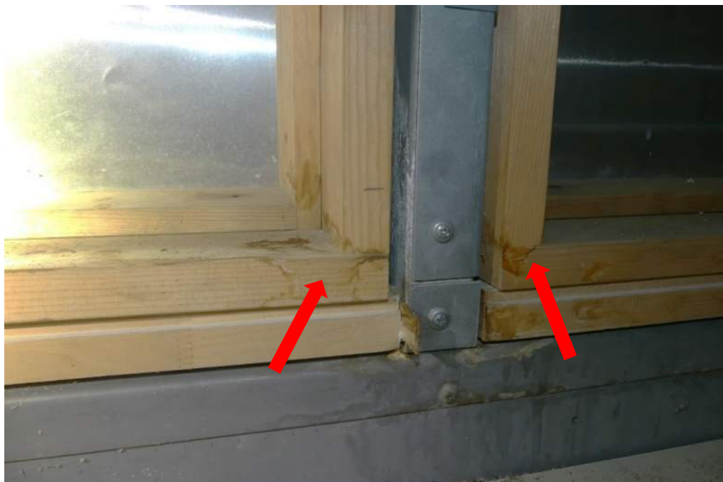
Photo 12 – Evidence of prior leaks on wood framing
