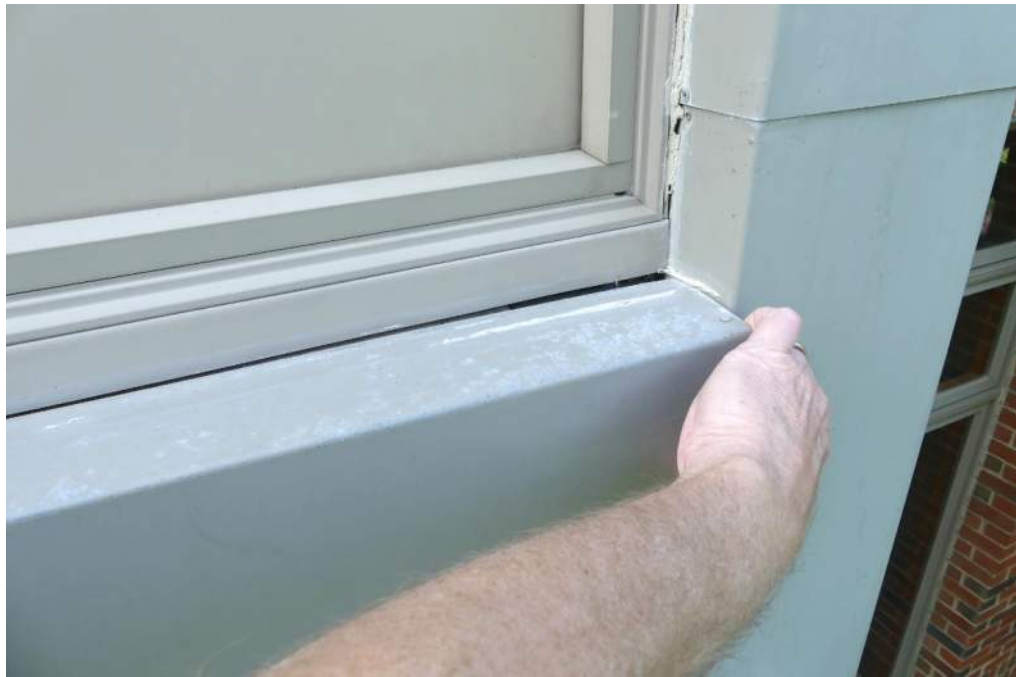
Photo 6 – Loose sill cover
