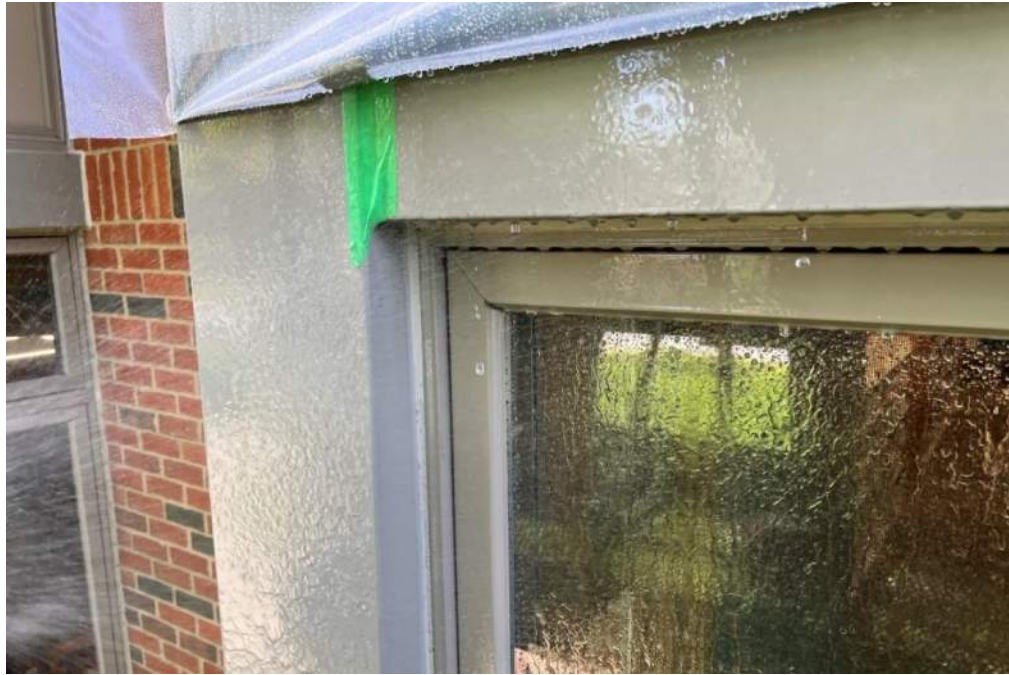
Photo 15 – Modified spray rack water test
