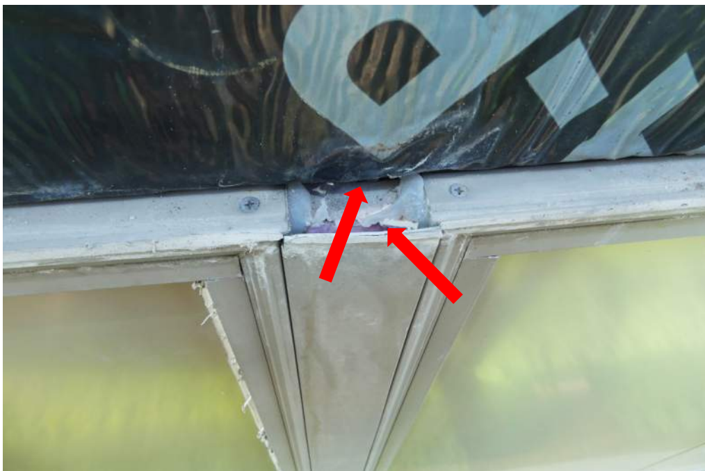
Photo 30 – Openings in top of mullion cap
