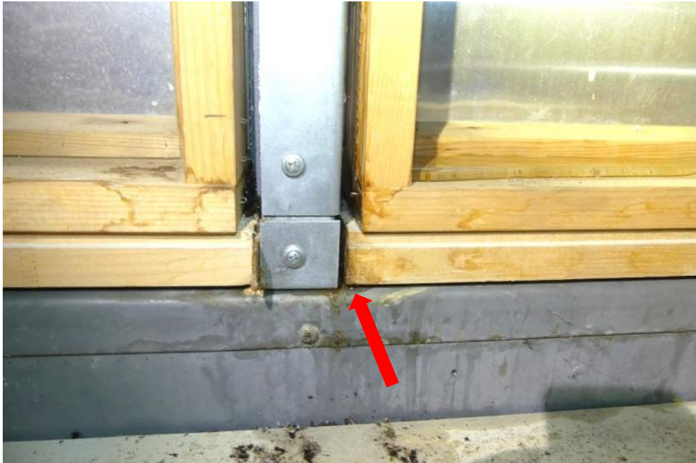
Photo 25 – Leak observed during test along 2 nd floor window sill
