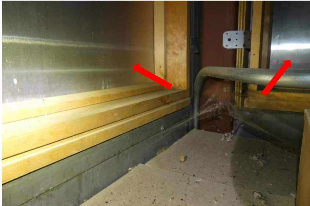
Photo 13 – No insulation or air barrier behind spandrel panels
