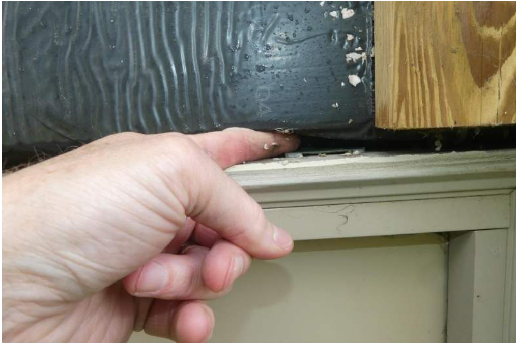
Photo 29 – Moisture in gap between flashing membrane and spandrel panel
