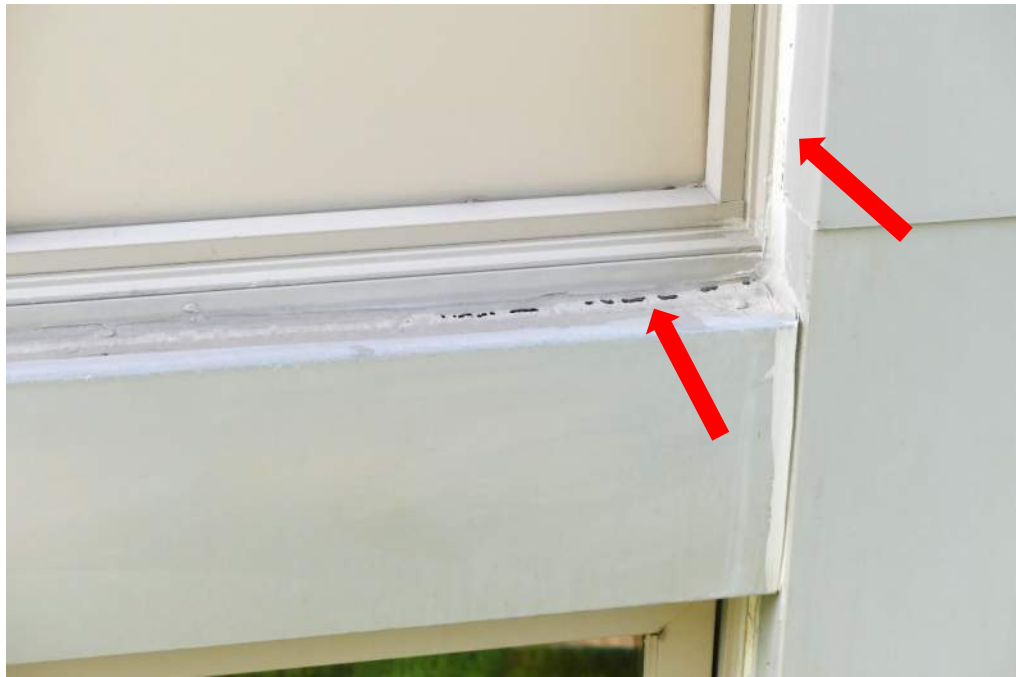
Photo 2 – Sealant exhibiting cohesive failure
