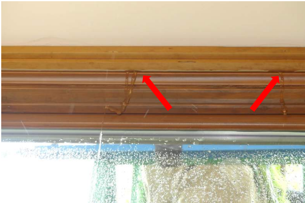
Photo 20 – Leak emanating between frame and trim
