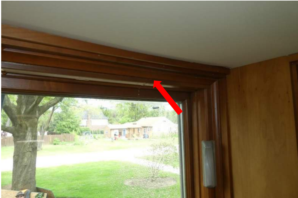
Photo 23 – Leak observed during test along 2 nd floor window sill
