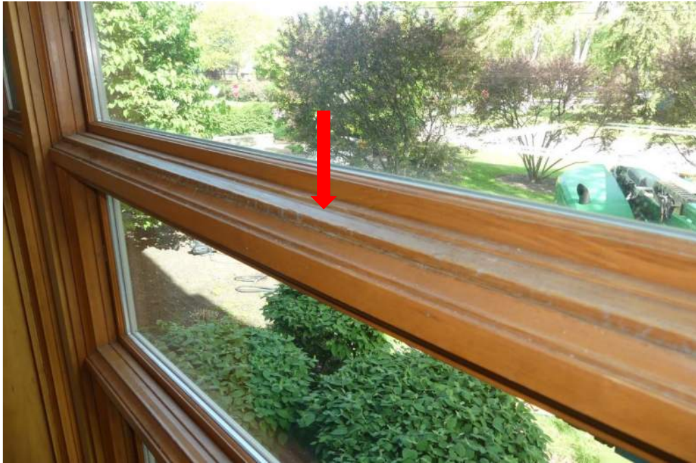
Photo 9 – Evidence of prior water leakage
